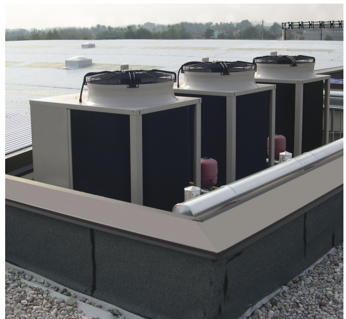
Fig. 2 - Robur GAHP-AR gas absorption heat pumps installed on roof with no need of boiler room.
